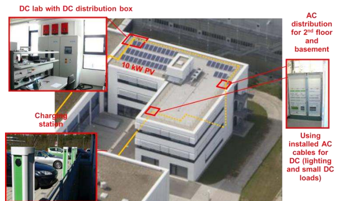
Figure 10: Fraunhofer Institute IISB building AE in Erlangen is the office test bed for proposed 380 V DC grid.
