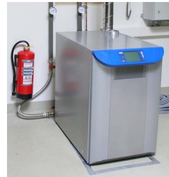
Fig. 5. MTT \mu -CHP unit installed in the offices demonstrator with gas supply
