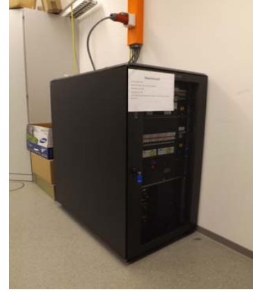
Fig. 4. Emerson Power Rack inside the DC laboratory, containing the grid controller, two 15kW rectifiers and the integrated MPPT-unit
