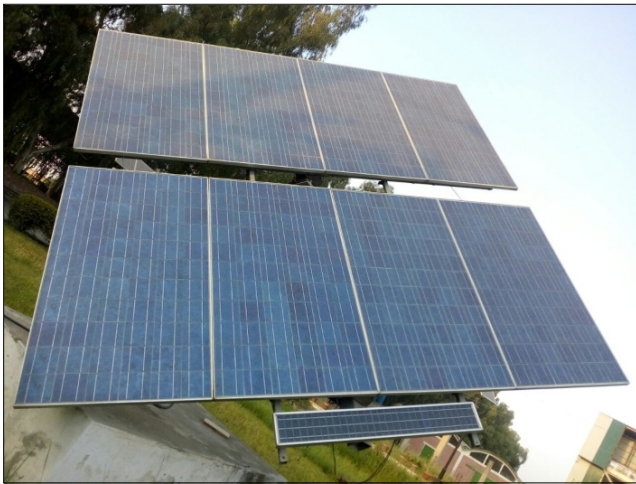
Figure 5. SPS with E-W single axis solar tracker
