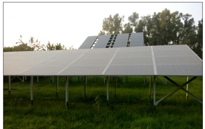
Figure 4. SPS with fixed angle mounting structure
