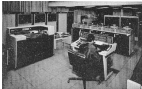
Figure 5. The CDC 3300 at ICA’s headquarters (circa 1970). The punched-card reader and magnetic-tape units are to the left, with removable disk units toward the back. Curtains in the front and back of the building were drawn to help control the temperature. Toward the top there is a glimpse of the mezzanine floor housing programmers. (Courtesy of Fundación ICA.)
