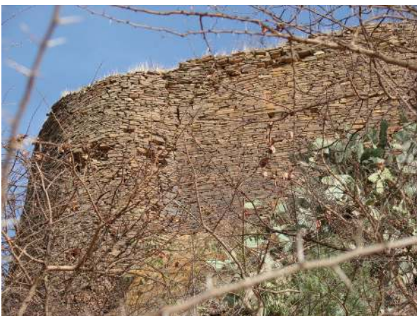
FIGURE 39. A detail of the dry stone masonry of the Fremona defensive walls and bastion. Photo by V.M. Fernández.
