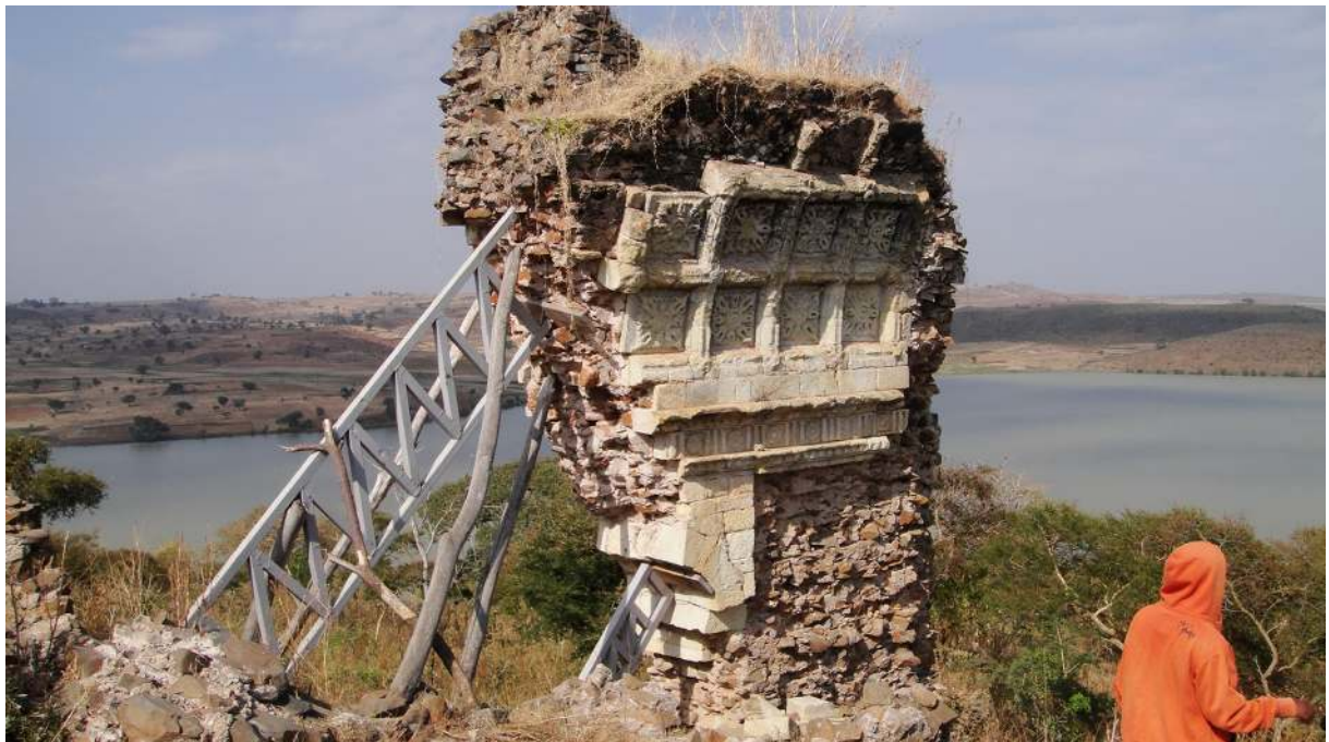
FIGURE 15. The apse of Gorgora Nova church after the protection scaffold was installed in 2009. Photo by V.M. Fernández.
