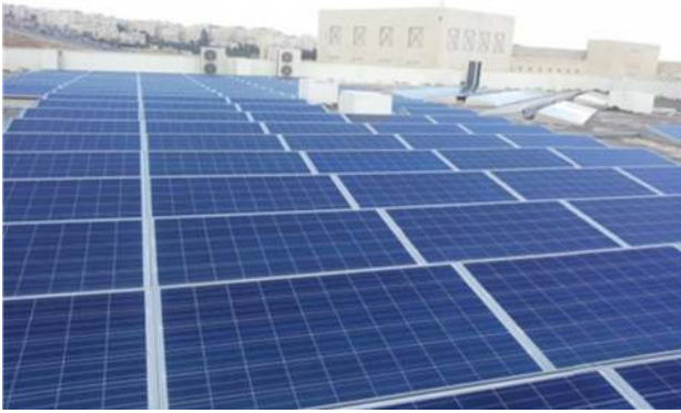
FIGURE 1. The 231 kWac PV system installed at the ASU, Amman, Jordan.
