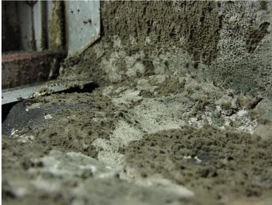
Figure 1. Typical example of a highly contaminated mechanical ventilation duct. Image courtesy of Total Ventilation Hygiene Pty Ltd and licensed for use in the HB2012 presentations and associated media.
