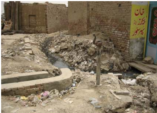
Figure 2: Blocked drains due to solid waste dumps.
