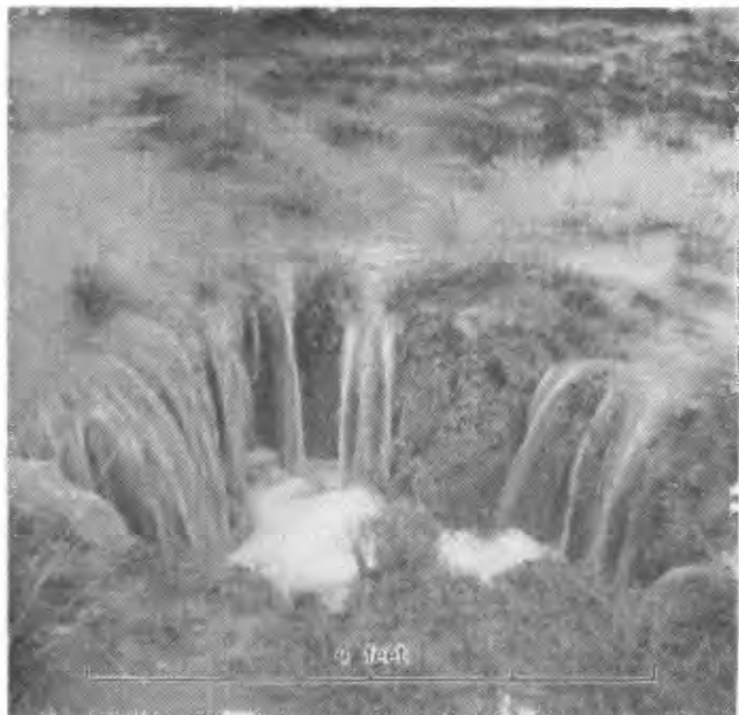
FIGURE 5.—Water pouring into open pipe or tunnel leading downward to arroyo channel. The upper opening of this piping hole is at least 15 feet from wall of gully. Rio Pescado near Ramah, N. Mex., August 17, 1946.
