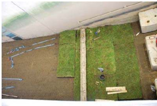
Figure 3.30 Installed grass sods including the underlying wooden plate and the steel hooks.
