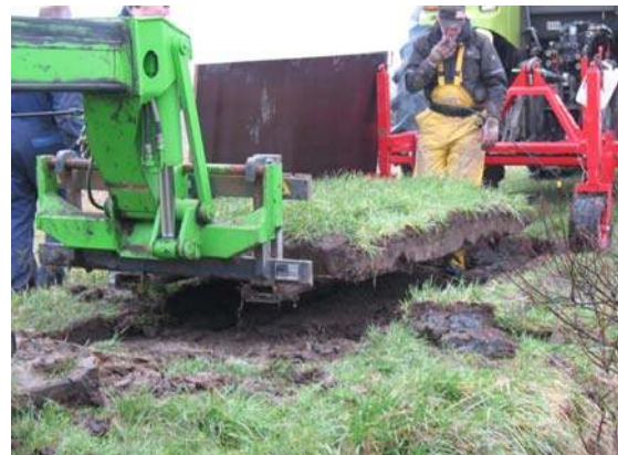
Figure 3.15 Lifting the grass sod on the wooden plate with a fork lifter.
