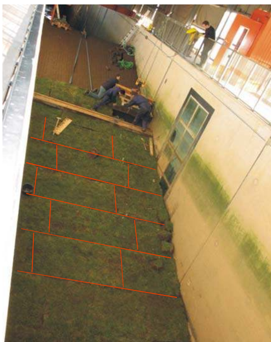
Figure 3.24 Displaced order on the seaward dike slope.
