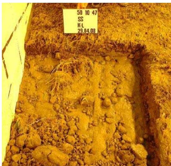
Figure 5.28 Damaged grass cover on the seaward slope during wave overtopping tests.
