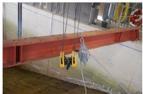
Figure 3.33 Crane hook, deflexion pulley and steel cable.
