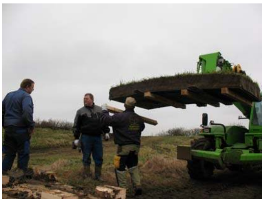
Figure 3.18 Installation of four wooden beams for further handling of the grass sods.
