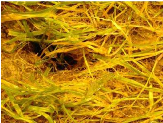
Figure 5.23 Open joint between two grass sods.
