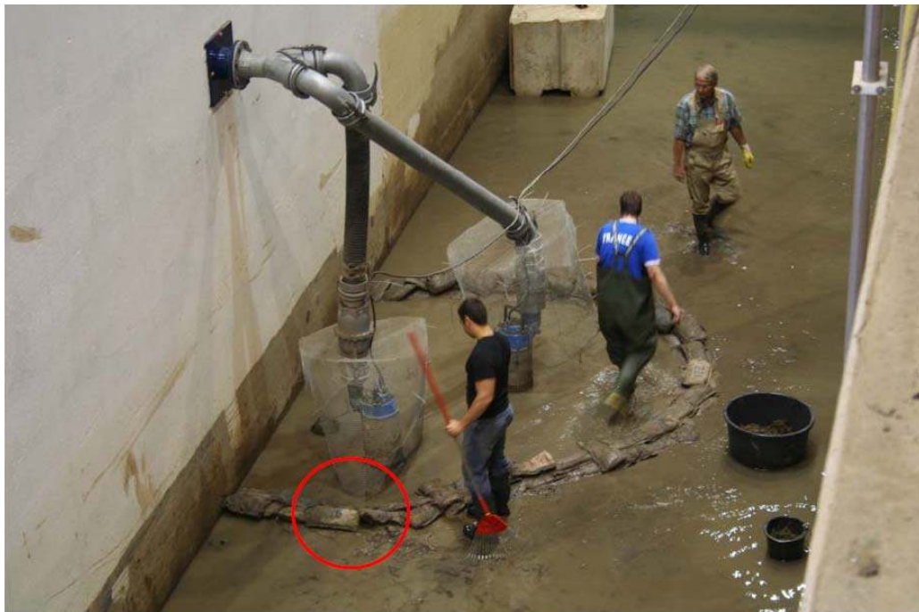
Figure 3.44 Two pumps on the landward side.
