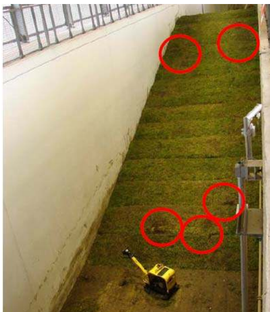
Figure 3.37 Damaged grass surface due to compaction.
