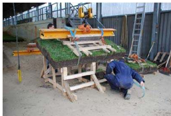
Figure 3.27 Tightening the grass sod to the transport frame and the steel beam with synthetic ropes.
