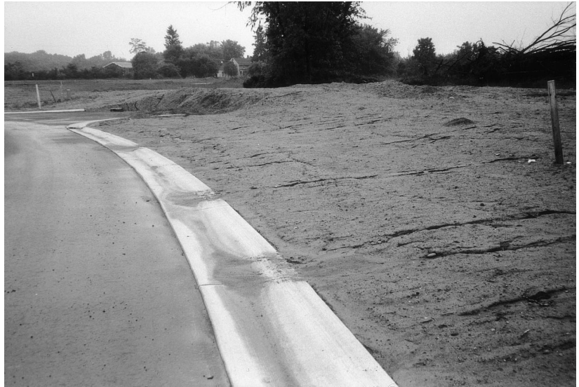
Figure 4. Inadequate slope stabilization.
