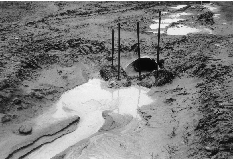
Figure 3. Improper water management.
