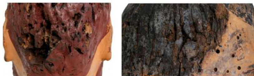
Figure 2. Wooden puppet heads (WPHs): deep deterioration of constitutive materials (left); flight holes 1.5–3 mm in diameter (right) related to the Anobium punctatum (de Geer 1774) infestation.
