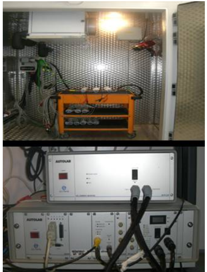
Figure 3: The climatic chamber and used measurement devices of battery impedance
