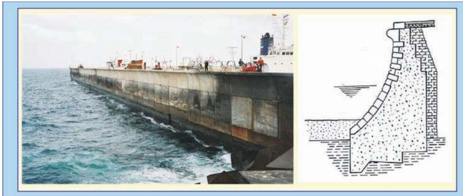
Fig. 7.17: An example of a modern, large vertical breakwater with wave return wall (left) and cross-section of an older seawall with recurve (right)
