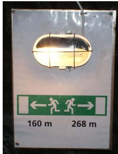
Figure 2. A picture of the emergency sign installed every eight meters inside the tunnel.
