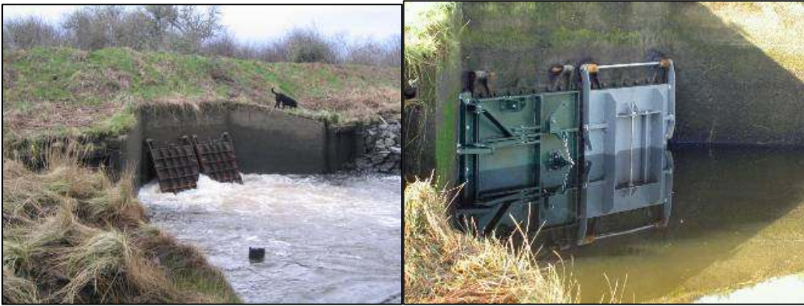
Figure 2.3. Tidegates at Vera Slough Before (left) and After (right) Replacement (photos courtesy of CREST)
