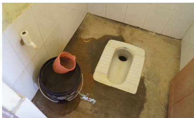
Figure S4. A typical latrine with a water bucket found in surveyed schools.
