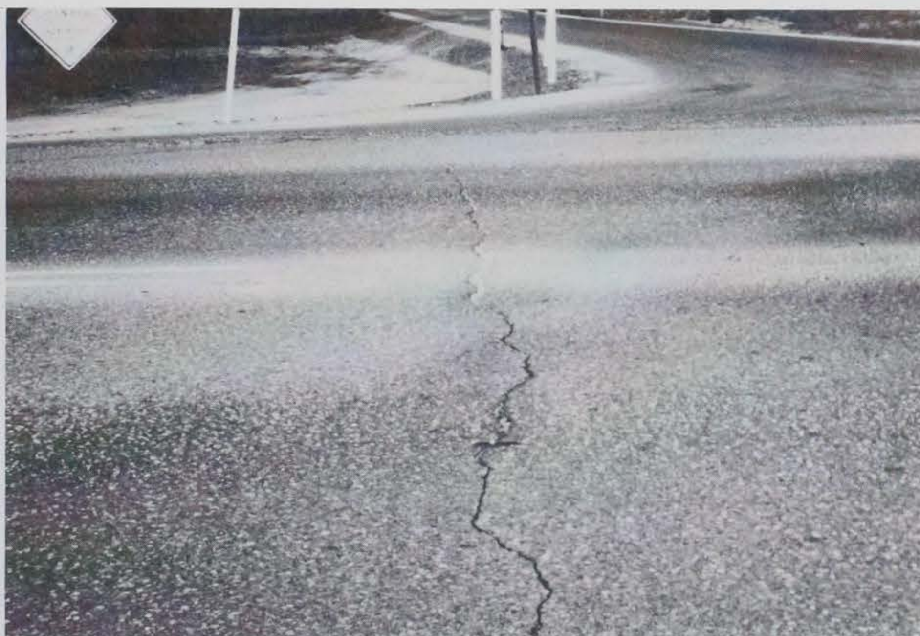
Figure 21. Typical transverse crack over original AC pavement, US 2, Spokane County
