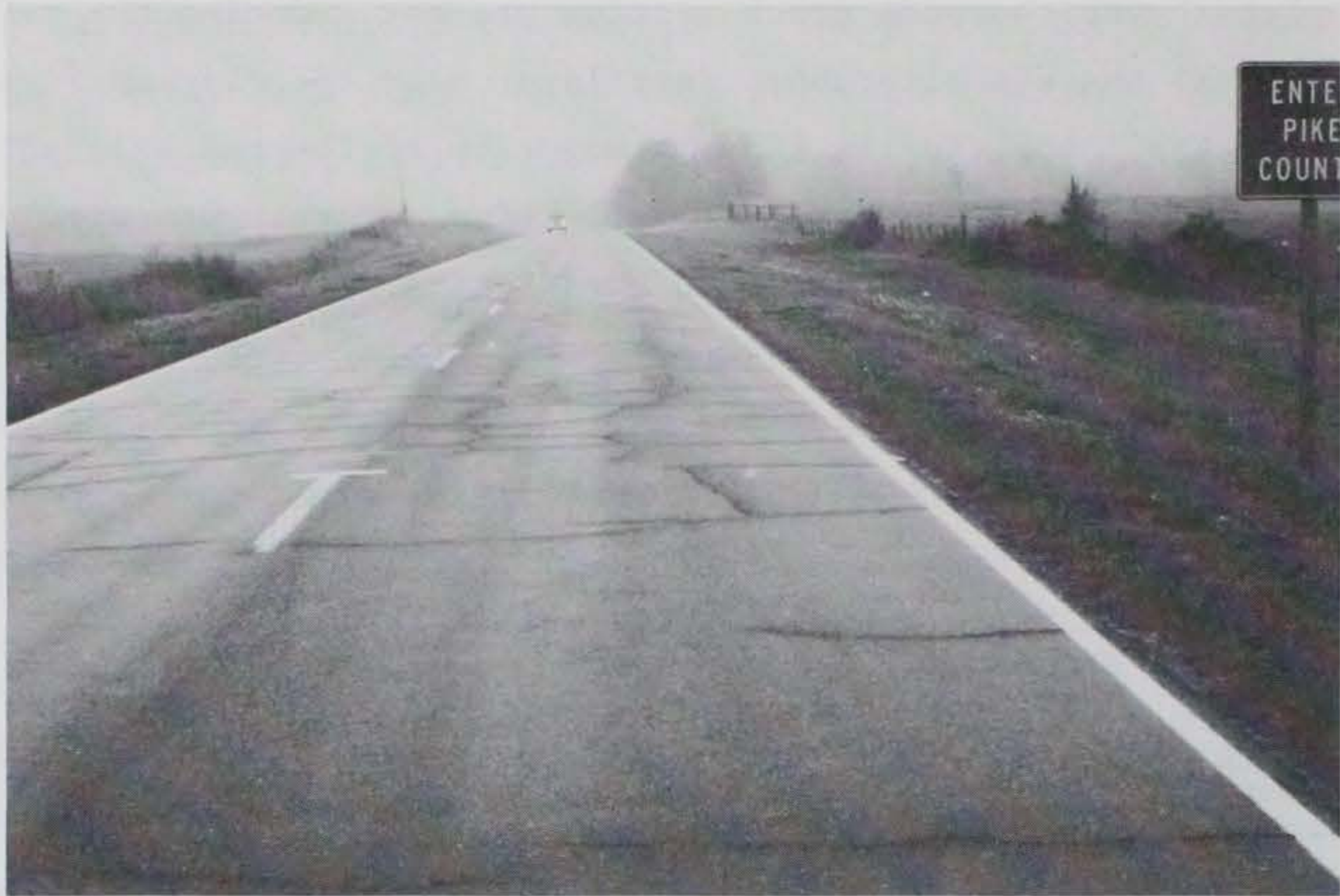
Figure 9. Comparison of asphalt-rubber interlayers, wide crack section (background), and slag seal section (foreground)
