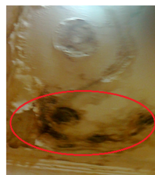
Figure 1: Site of S. chartarum isolation (wet wall).
