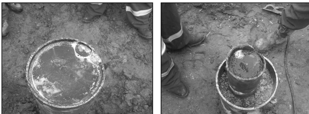
Fig. 7—Illustration of leaking casing caps found at wellbore re-entry on surface casing and production casing.
