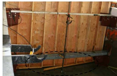
Fig. 10. Failed bottom plate of TW 1 (unanchored, Specimen 1A)
