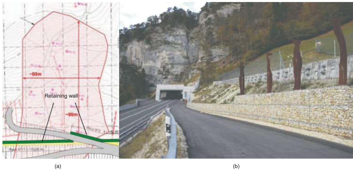
Fig. 5. Northern part of Combe Chopin landslide: (a) schematic outline of landslide; (b) photograph of wall (courtesy of Stump)
