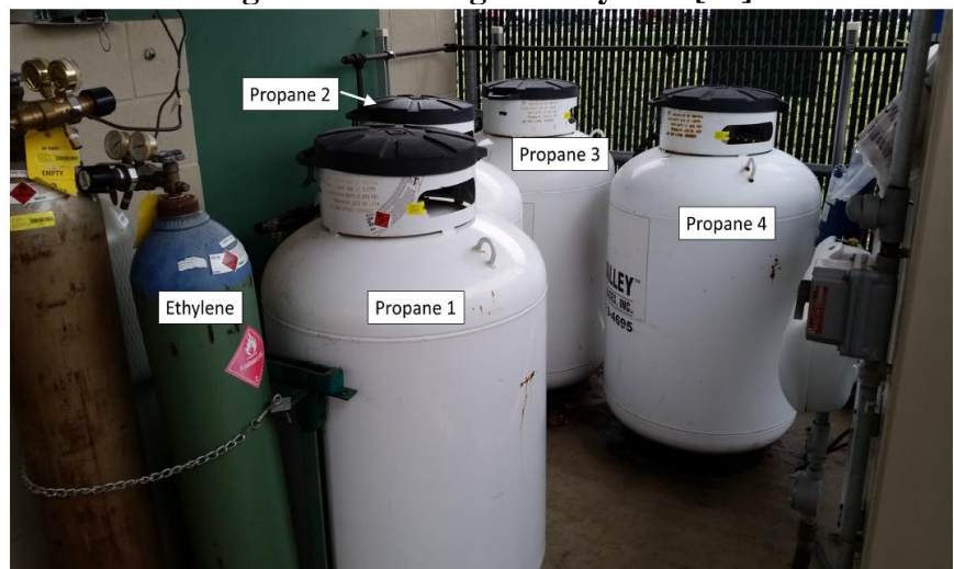
Figure 50: COAL lab fuel facility [33]
