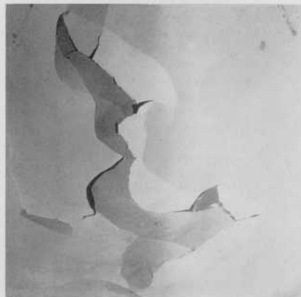
FIGURE 2. Bulging of white coat on a side wall, involving separation of the finish (or white) coat from the sanded gypsum base coat within an area of about 1 sq yd.
