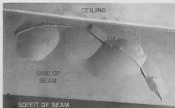
FIGURE 1. Bulges in white coat along the side of a concrete beam, caused by the expansion attending the slow hydration of free MgO present in the hydrated lime used in preparing the white coat.
