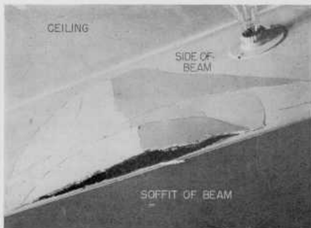
FIGURE 14. Plaster failure involving the expansion of about 0.5 percent in the white coat along the side of a concrete beam.
