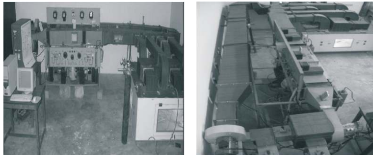
Figure 3. Photographic view of FLC based VRV-VAV A/C system
