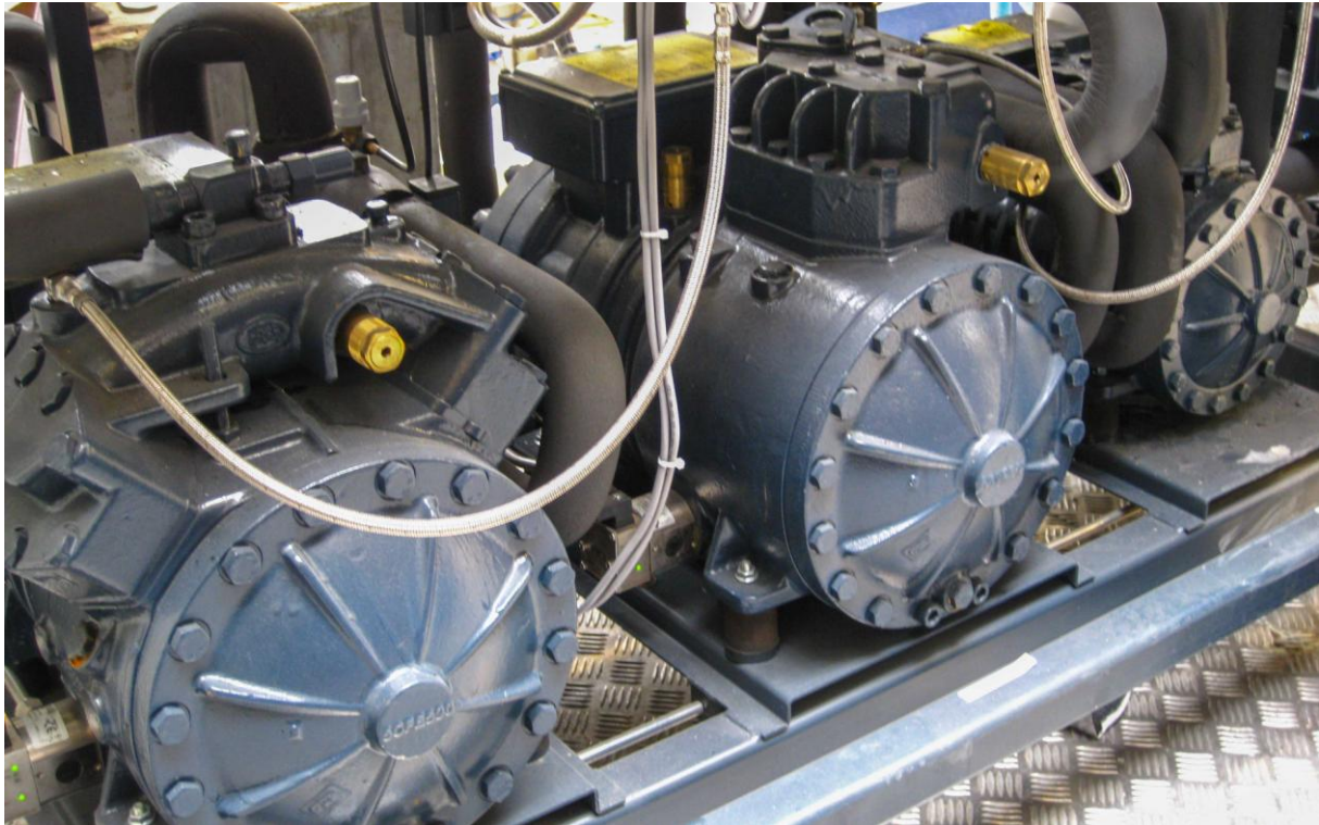
Figure 5.4: The rack of the piston-type R744 compressors. On the left: base-load Dorin CD1400H, parallel #1 Dorin CD1000H, and parallel #2 Dorin CD380H.
