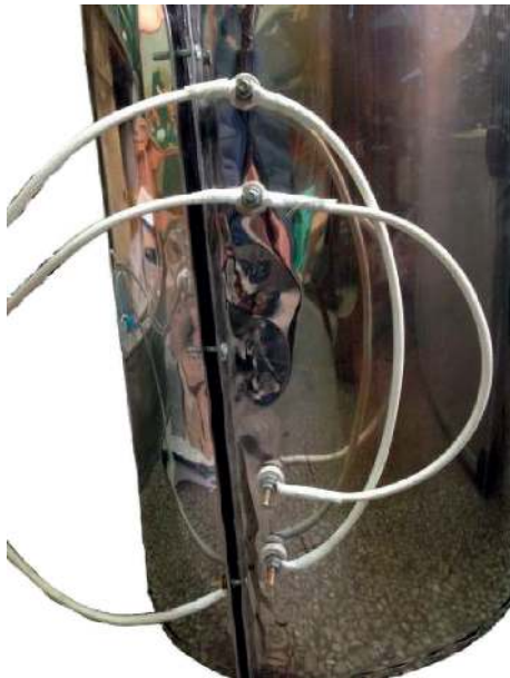
FIGURE 6: Electric heating equipment and interstar connection.
