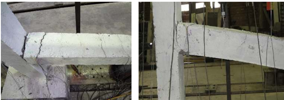
FIGURE 7: Crack pattern in south end of the specimen.
