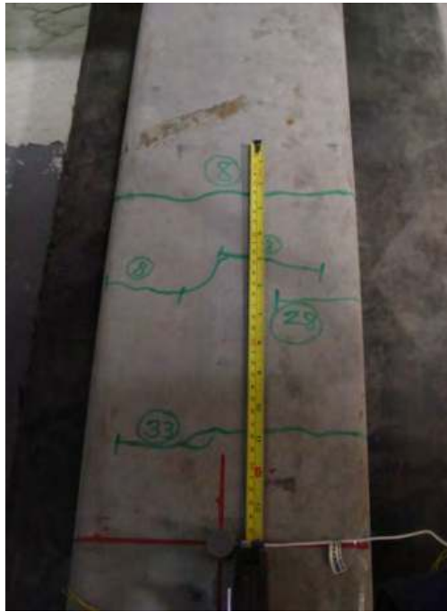
Figure 8.23 Cracks in a sleeper mid-span in hard track after 50 drops of 740 kN
