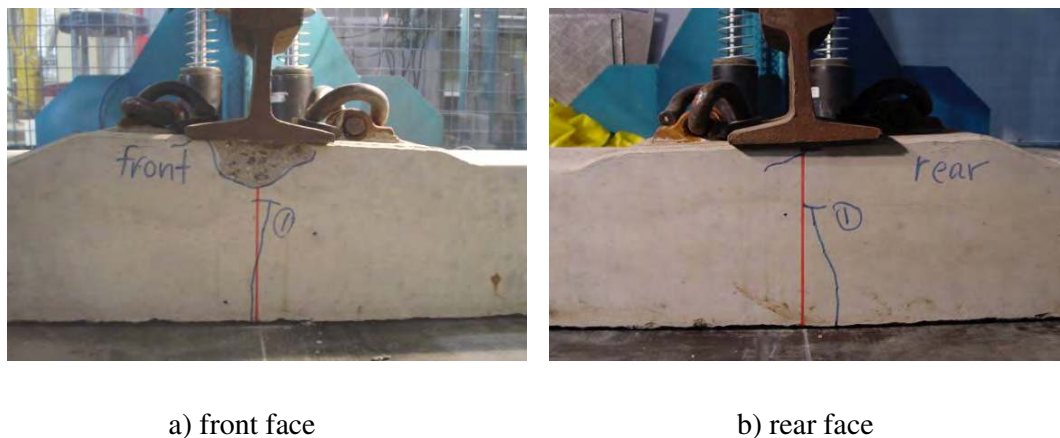
Figure 8.11 Cracks in a sleeper in hard track after a single impact of 810 kN
