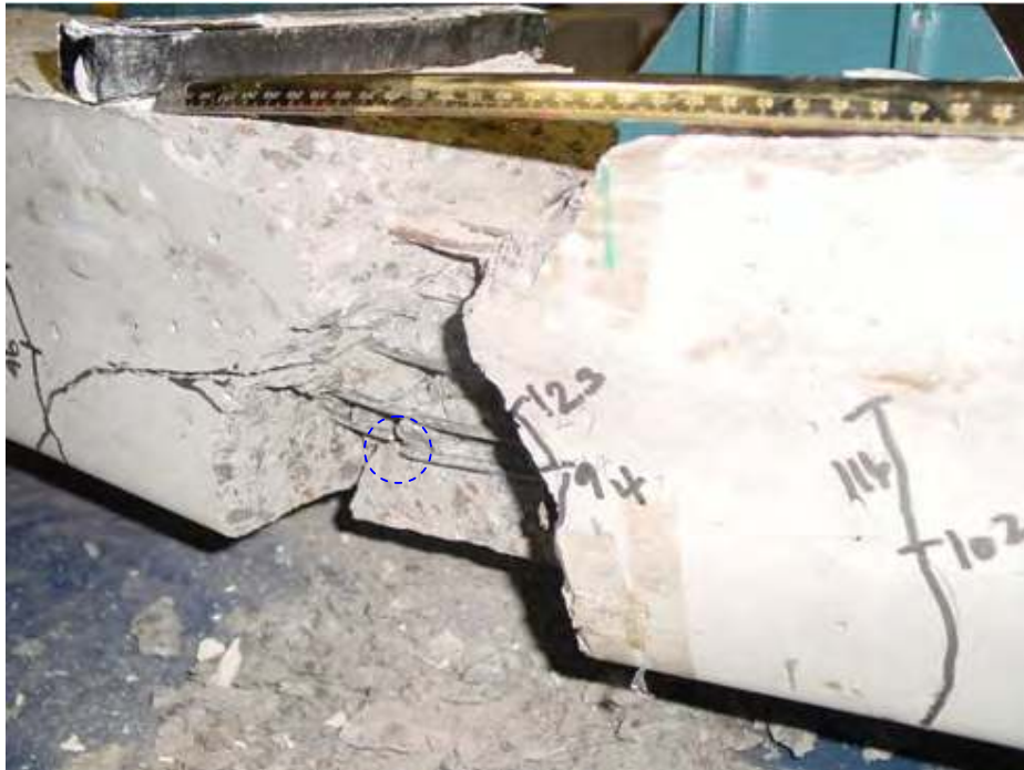
Figure 5.17 Damage of the lowest-layer prestressing wires of AUS-BG Sleeper
