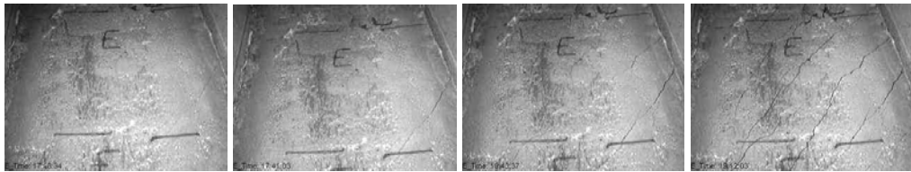
Figure 15: Retrofitted pier PO2 damage from internal east side view.
