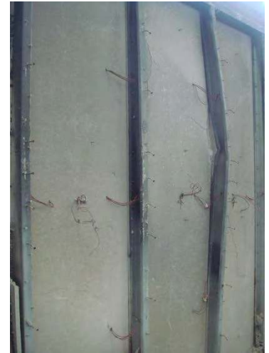
(c) Steel frame after fire
