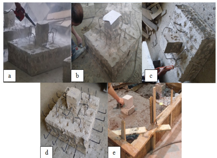
Figure 8: Preparation process (a) Roughening the concrete surface. (b) Drilling. (c) Installing epoxy. (d) Installing and placement dowels. (e) Casting new jacket.
