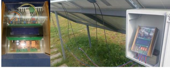
Figure 4. Photo of the electrical measurement device.
