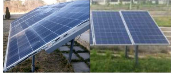
Figure 2. PV panels placed with an optimum annual angle of 34°.
