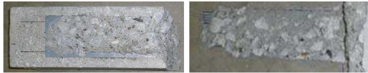
a. failure within concrete substrate (B-1 series)
