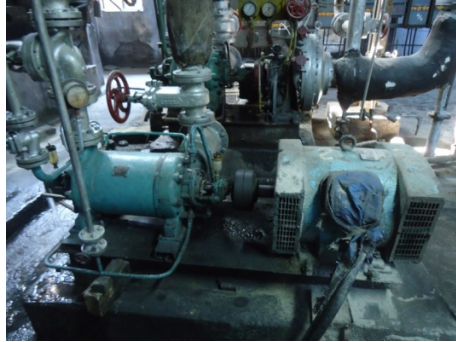
Fig. 15. Photograph of boiler feed pump
