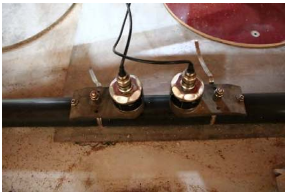
(a) Two sensors connected to pipe
