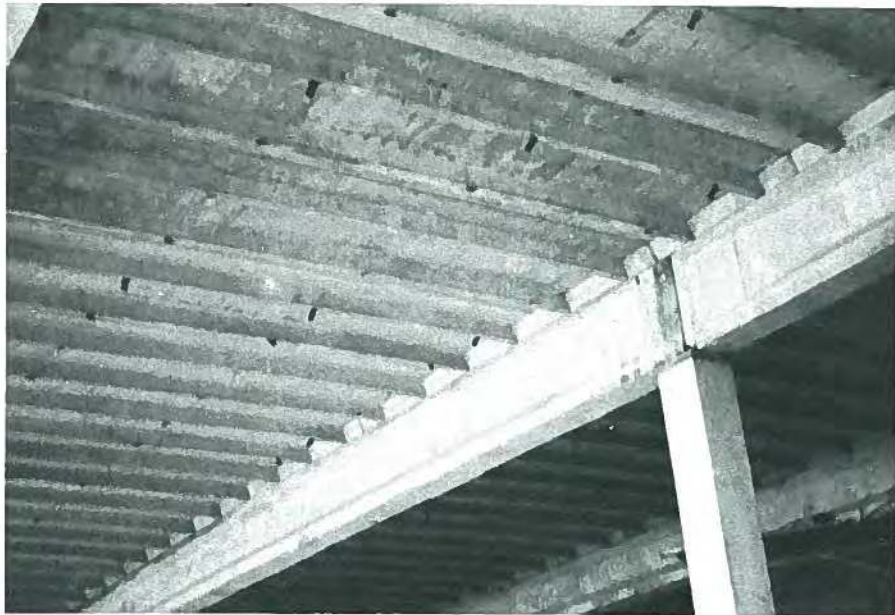
Fig. 10. A 6-ft (1.83 m) wide double-tee was developed from existing channel slab designs to allow larger spans between beams in the cold storage warehouse for Beatrice Foods.
