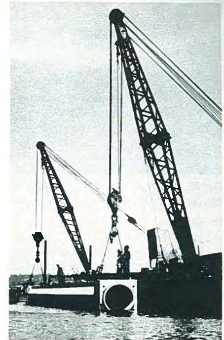
Fig. 87. 85-ton (77 t) precast prestressed hollow pipe section being installed in Lake Washington.
