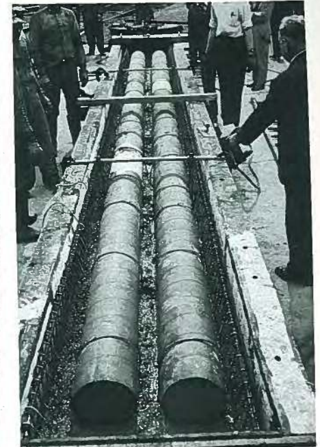
Fig. 20. Girder is about half cast, showing paper tubes used to form voids in the concrete.
