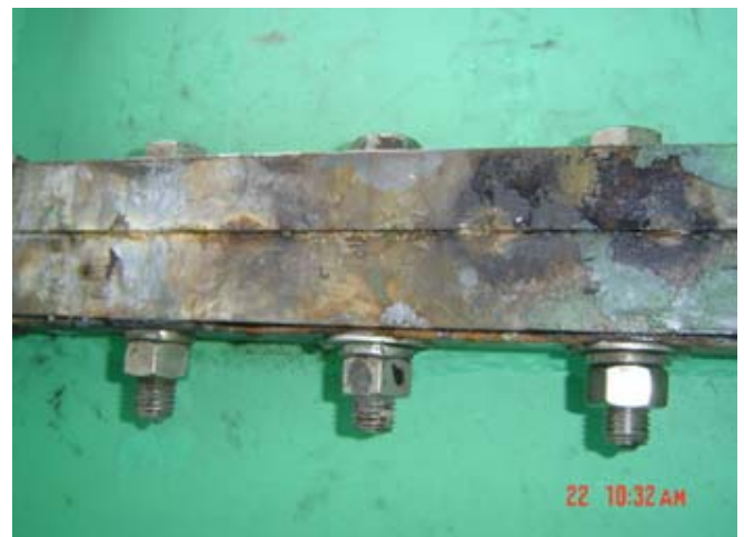
Fig. 3. Paint loss due to overheating in the connection of flange-screws (front view).
