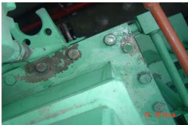
Fig. 4. Paint loss due to overheating in the connection of flange-screws (top view).
