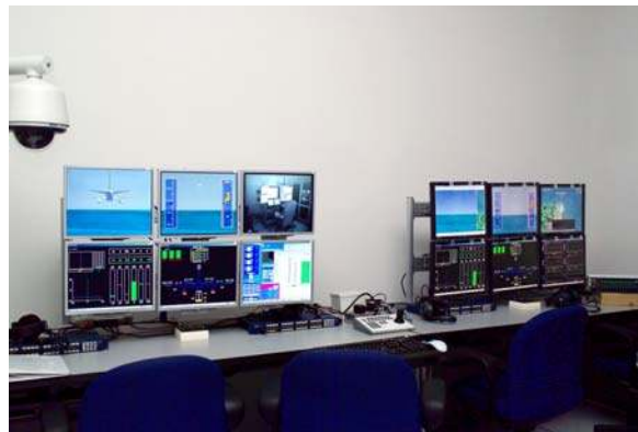
Figure 10. Photograph of Operations Command Station and Operations Engineering Stations in BRS
