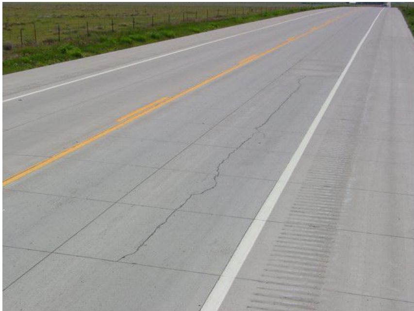
Figure 2.15 Typical Cracked Slab Conditions Observed at the U.S. 287 Lamar Site (Sheehan et al. 2004)
