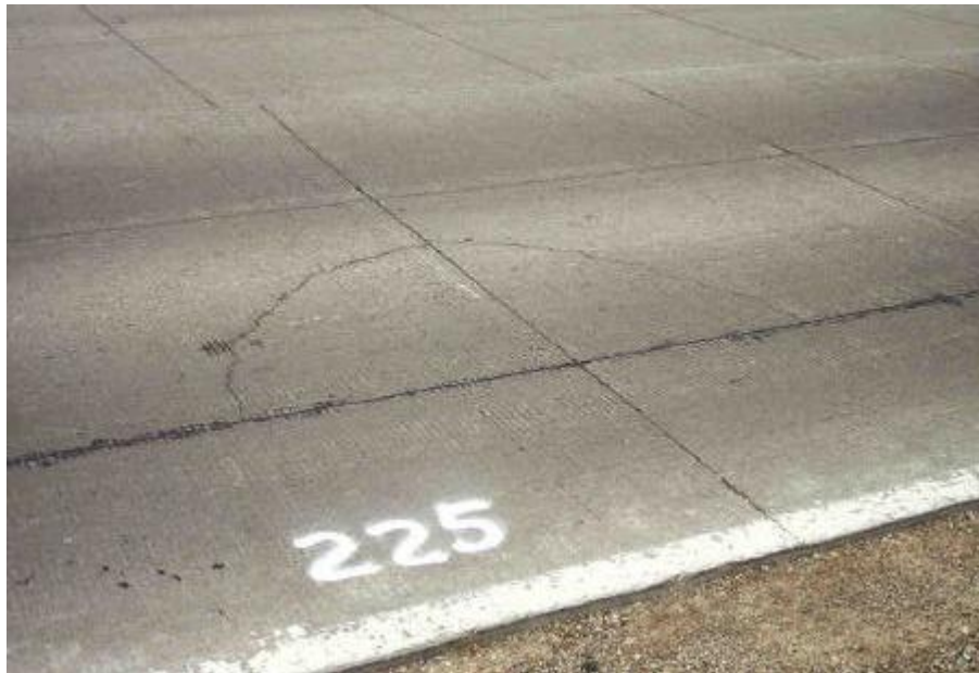
Figure 2.16 Panel Corner Breaks in Tuscola Project (Winkelman 2002)
