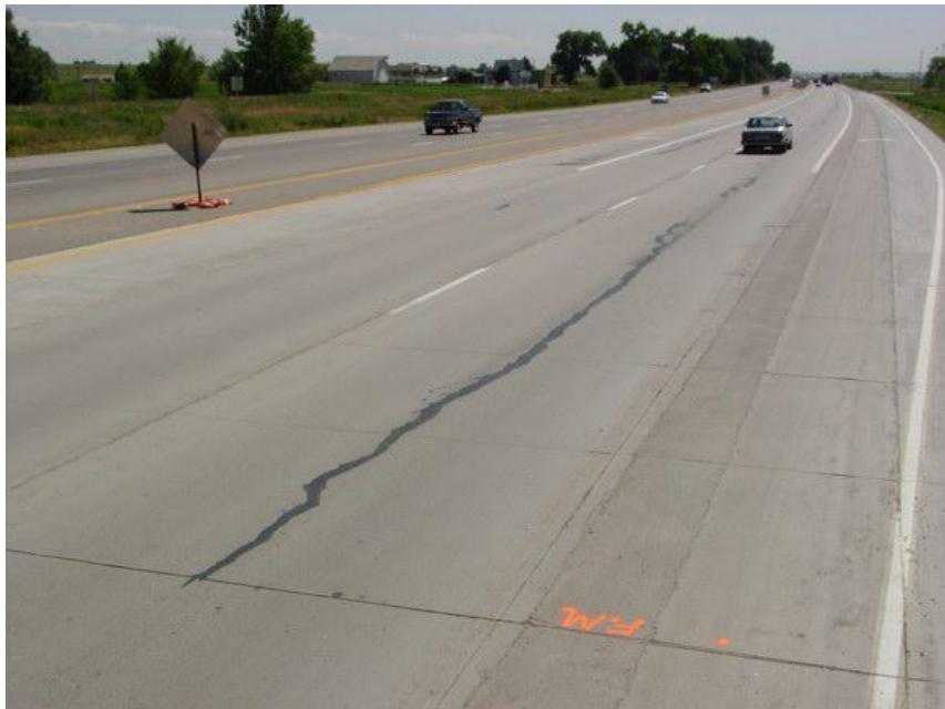
Figure 2.13 Typical Slab Cracking Observed in S.H. 119 Test Section No. 2 (Sheehan et al. 2004)
