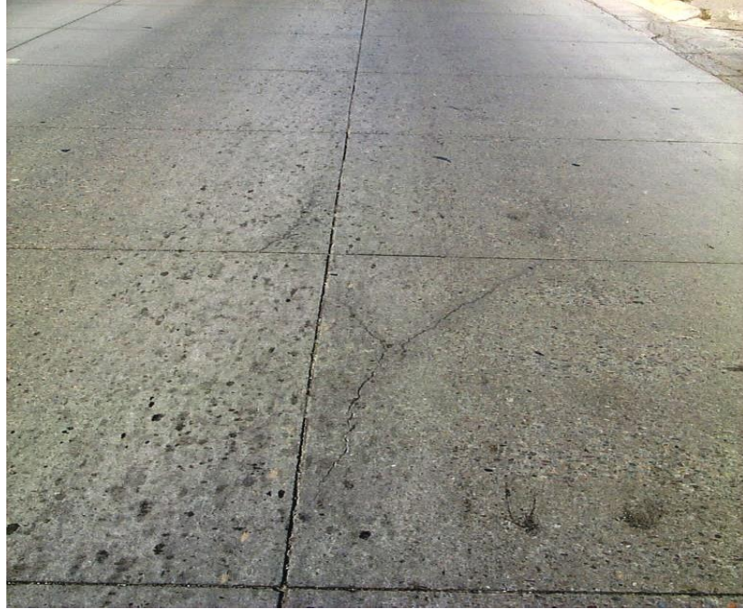
Figure 2.17 Hairline Crack in Kalispell Project Pavement (MtDOT 2008)
