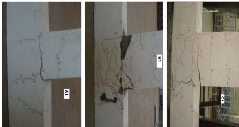
Figure 21. Crack pattern of group-I (A1, B1, C1).
