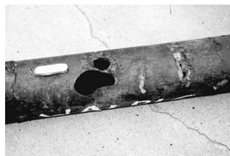
Fig. 5 Pipeline that experienced stray current corrosion caused by inverting the electrical leads to a cathodic protection rectifier
