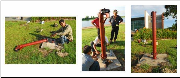
Base of the column is welded and the column being set up
