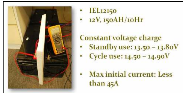
Figure 21. The battery bank.
