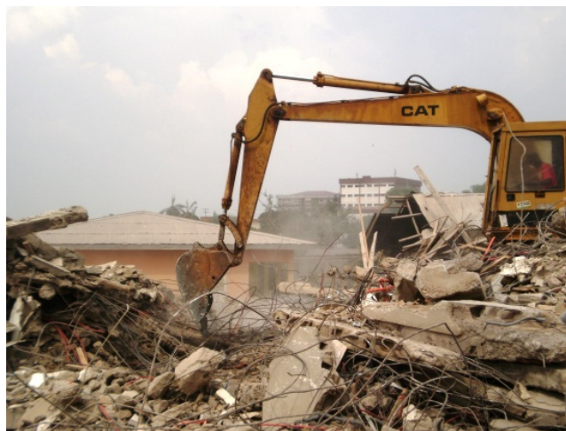
Figure 10. Collapse site of a 5-storey building at Nkoldongo, Yaoundé (Source: Journal du Cameroun, 2010)
