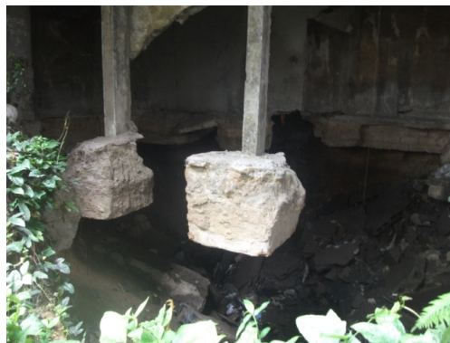
Figure 12. Foundation failure due to Erosion (Source: Author, 2014)
