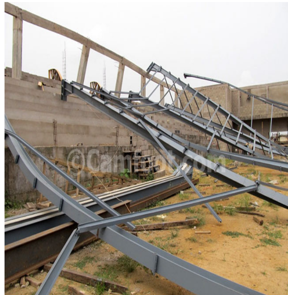
Figure 2. Multi-Sport Complex Steel Truss Roof collapse at Bépanda Suburb, Douala
