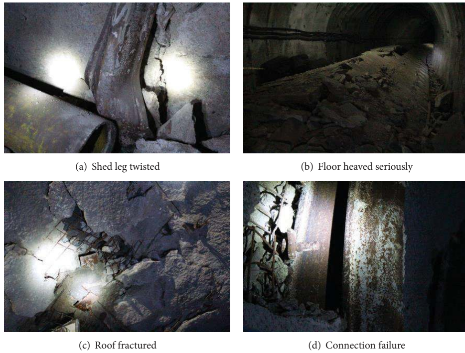
FIGURE 4: Deformation and failure of the roadway after repairing.
