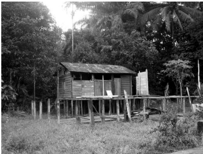
FIGURE 2 House damaged in 2006 flood in Paya Seturan village
