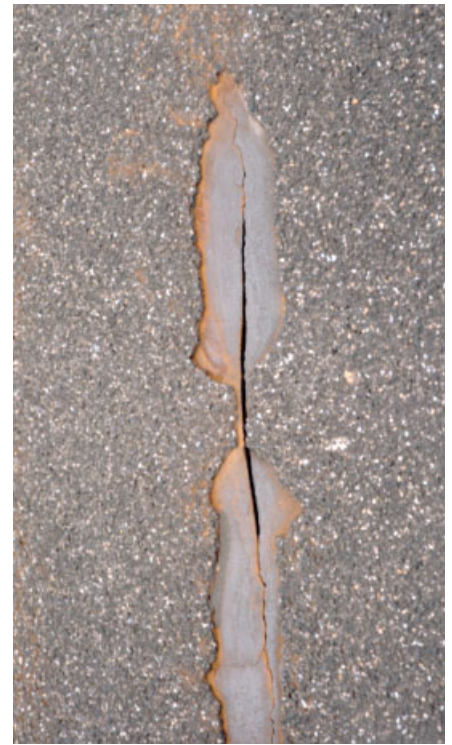
Fig. 3. Typical through-crack in deck plate (surfacing = 6 mm epoxy)
