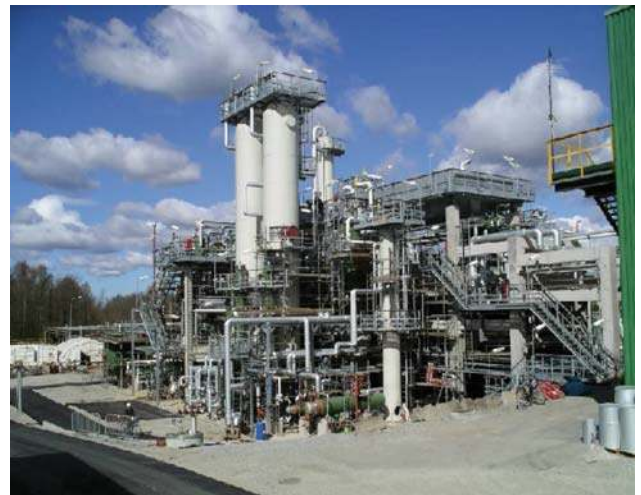
Picture 3 Perstorp 160 000 tpy plant (Sweden).
