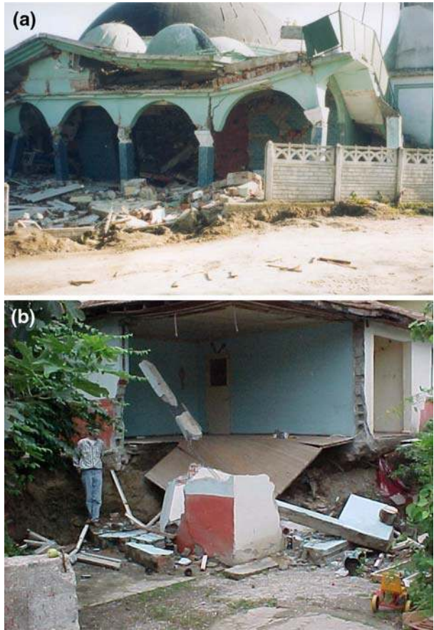
Fig. 15 Normal fault east of Gölcük, Kocaeli, Turkey 1999 earthquake—Denizevler: a Mosque resting on flexible foundation (isolated footings), and b 1-story cinder-block building (photo from Youd et al. 2000), directly founded on the ground (very flexible foundation). Both buildings were subjected to about 1.5 m differential displacement and partially collapsed
