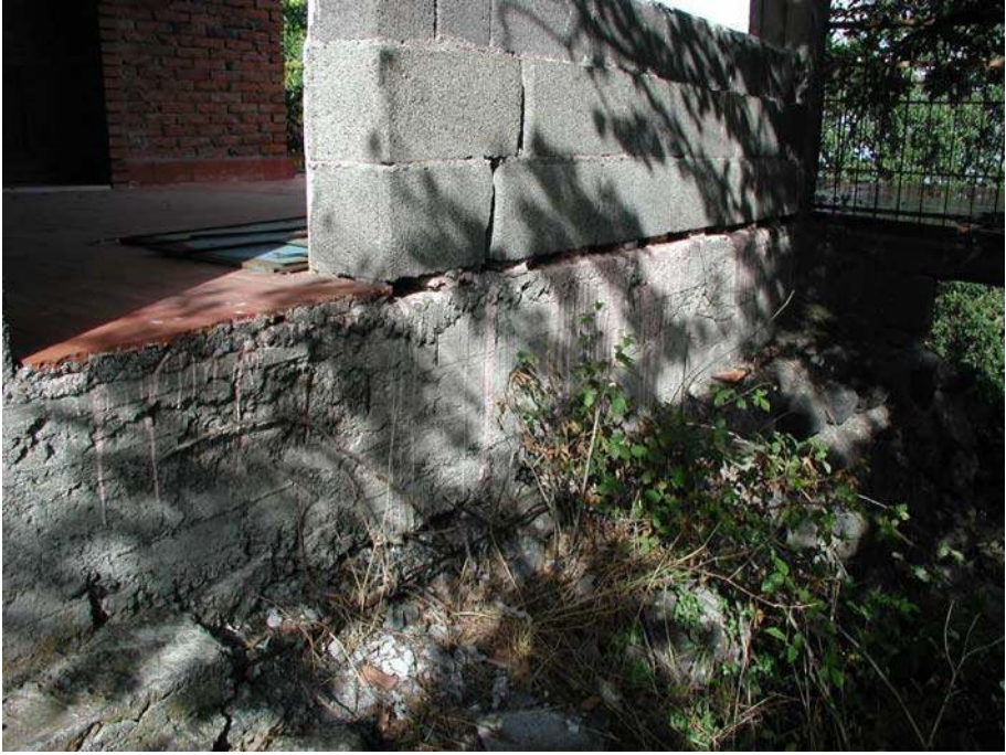
Fig. 5 Mt. Etna—1-story building of Fig. 4. Detail of the reinforced concrete ring beam around the raft foundation
