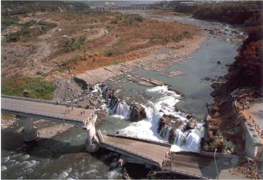
Fig. 19 Chelungpu thrust fault, Chi-Chi, Taiwan 1999 earthquake—Fung-Yan City. The fault rupture passed through the south abutment of the Bei-Fung bridge with an upthrust of about 7 m, causing the collapse of two spans and the development of a small, but impressive, waterfall (photos adapted from Hwang 2000 )
