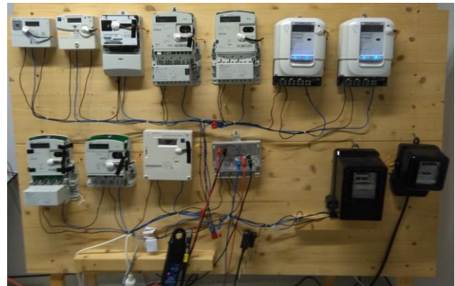
Fig. 1. Picture of the ten static meters placed in series, the energy meter reading of the static meters is corrected with the consumed energy of the following static meters
